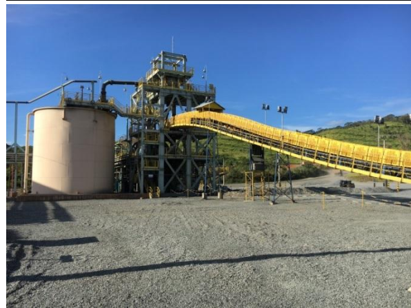
Figure 4: Ball mill and slurry storage tank
